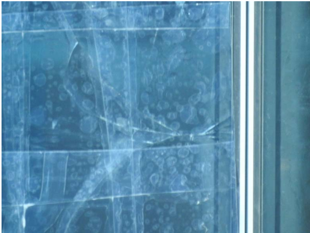
CLOSE-UP OF THE GLAZING CRACK AND SECURITY FILM INSTALLED
